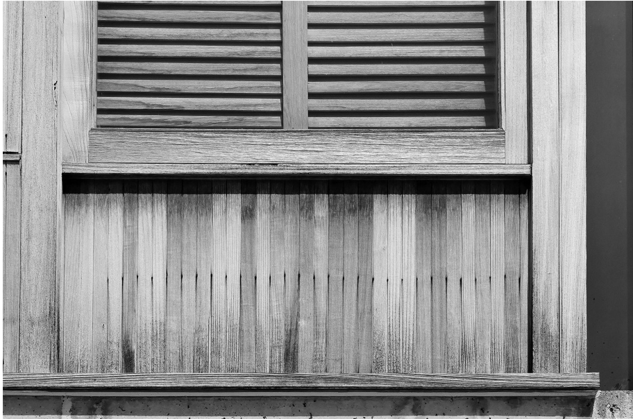
Figure 1. Louis I. Kahn, Salk Institute for Biological Studies, La Jolla California, 1963, weathered timbered cladding. Photograph by D. Leatherbarrow.
