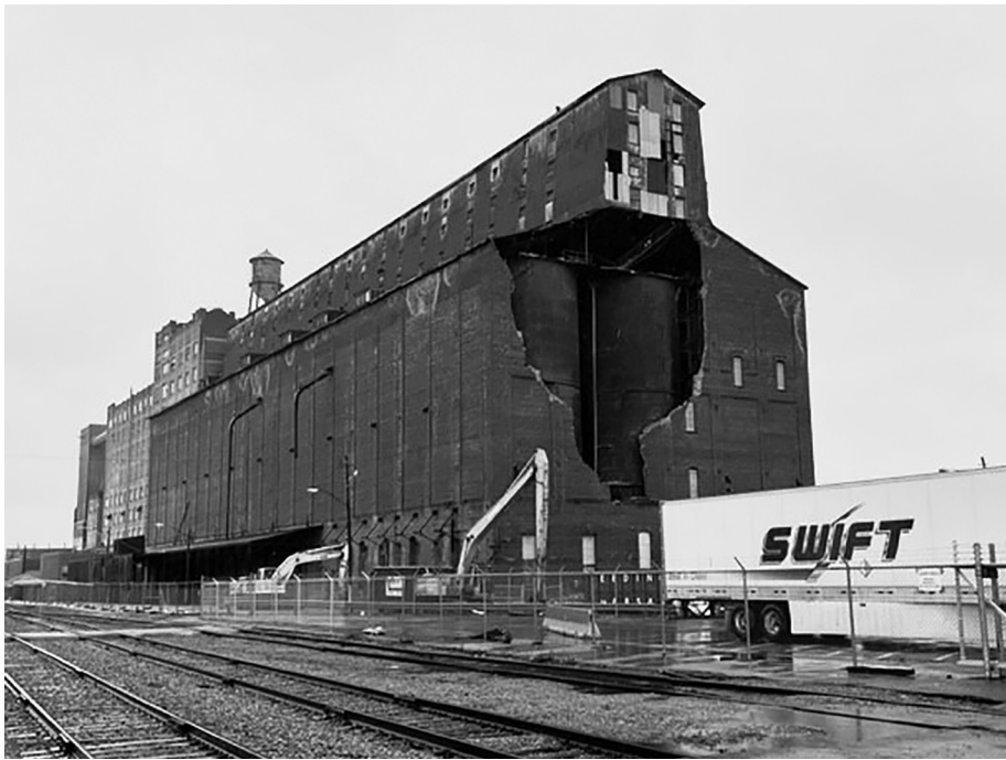
Figure 3. The Great Northern grain elevator. Photograph taken by C. Korsmeyer, December 2021. The interior silos can be seen through the hole caused by wind damage.
